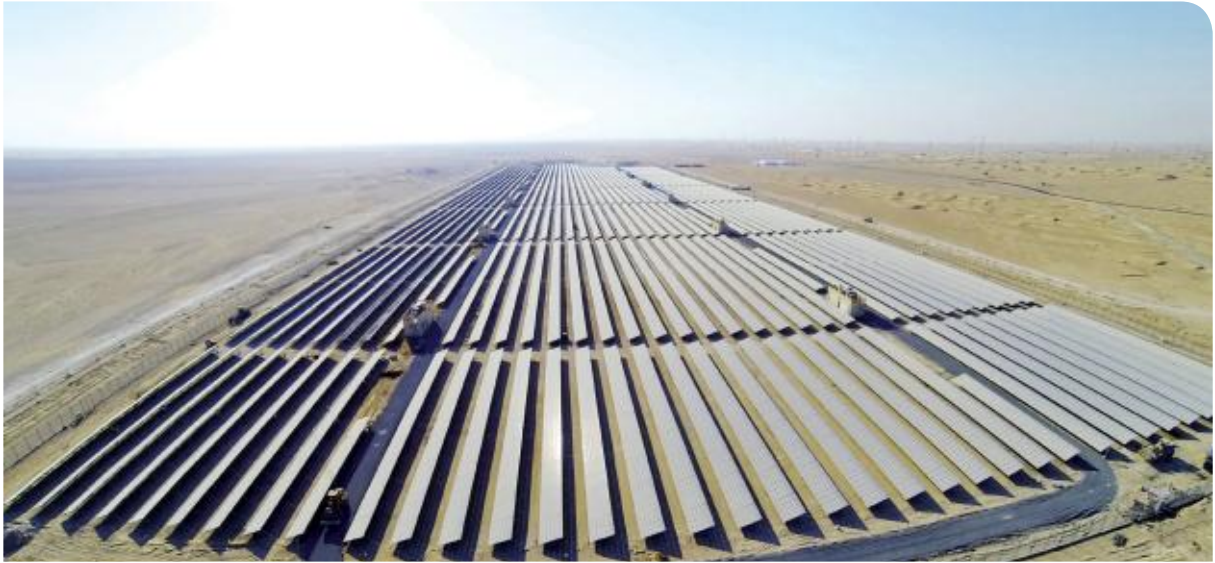
The third phase of Mohammed bin Rashid Al Maktoum Solar Park is expected to start operations in 2020
